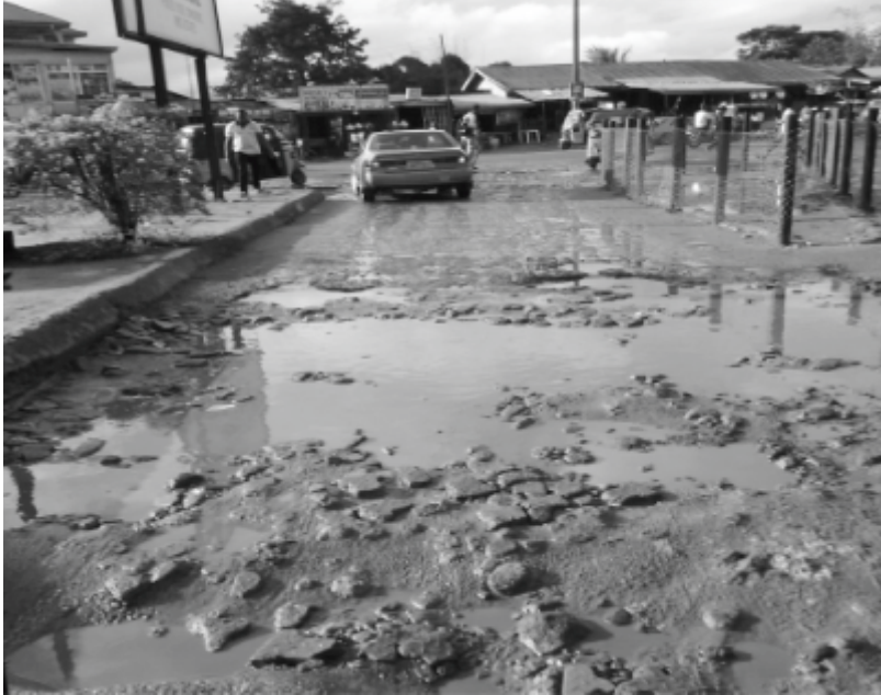
Plate 2: Showing the State of Road Near Polytechnic- FUTO Road Junction
