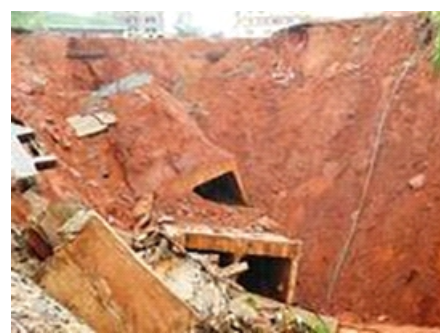
Plate 2: The effect of deep gullies that have damage major portions of the road at Ngwo
