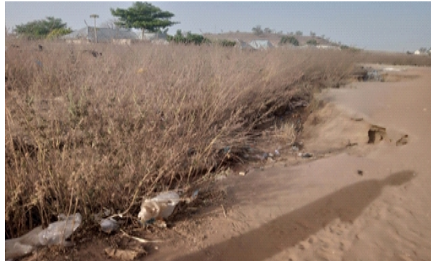
Figure 3: A damaged road beside UBE primary school, old Kwangwara (Site B)
