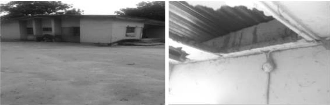
Plate 4: A Unit of Staff Quarters Ravaged By Termites with Possible Colonies in the Roof
