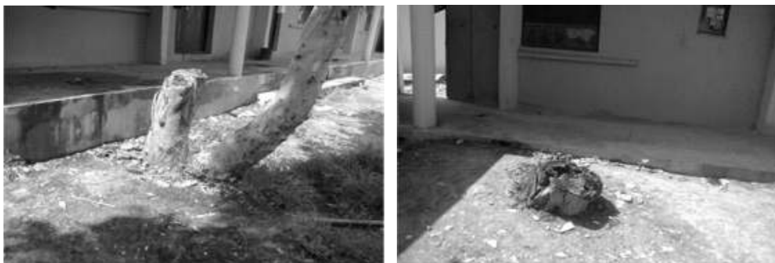
Plate 2: Stumps, Cutaway Tree, & Broken Blocks Forming A Hiding Place for Termites
