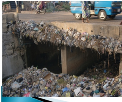
Plate 6. River channel blocked by waste at Rasco Area of Osogbo in the dry season Source: Authors Field Survey, 2019
