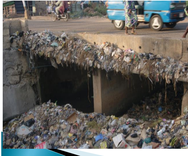
Plate 6. River channel blocked by waste at Rasco Area of Osoogbo in the dry season. Source: Authors Field Survey, 2019
