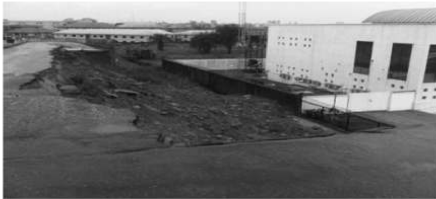
Picture 1: Collapse of 10-year old bridge in Port Harcourt, September 2012 Source: Field Study (2012).
