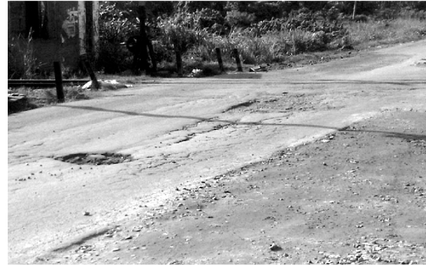
Plate 2: Shows a pothole at the railway line road before Inisha town
