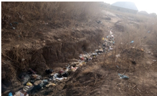
Figure 4: A damaged road beside FCE Kontagora fence (Site C)
